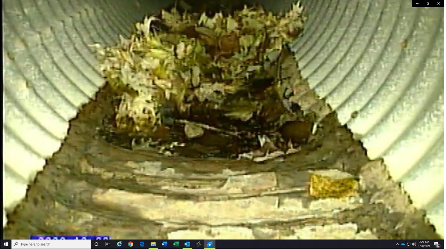
Attachment: Culvert Failure (RESOLUTION 3807 : Acquisition of Drainage Easement & Awarding a Culvert Replacement Project at 9731 N
