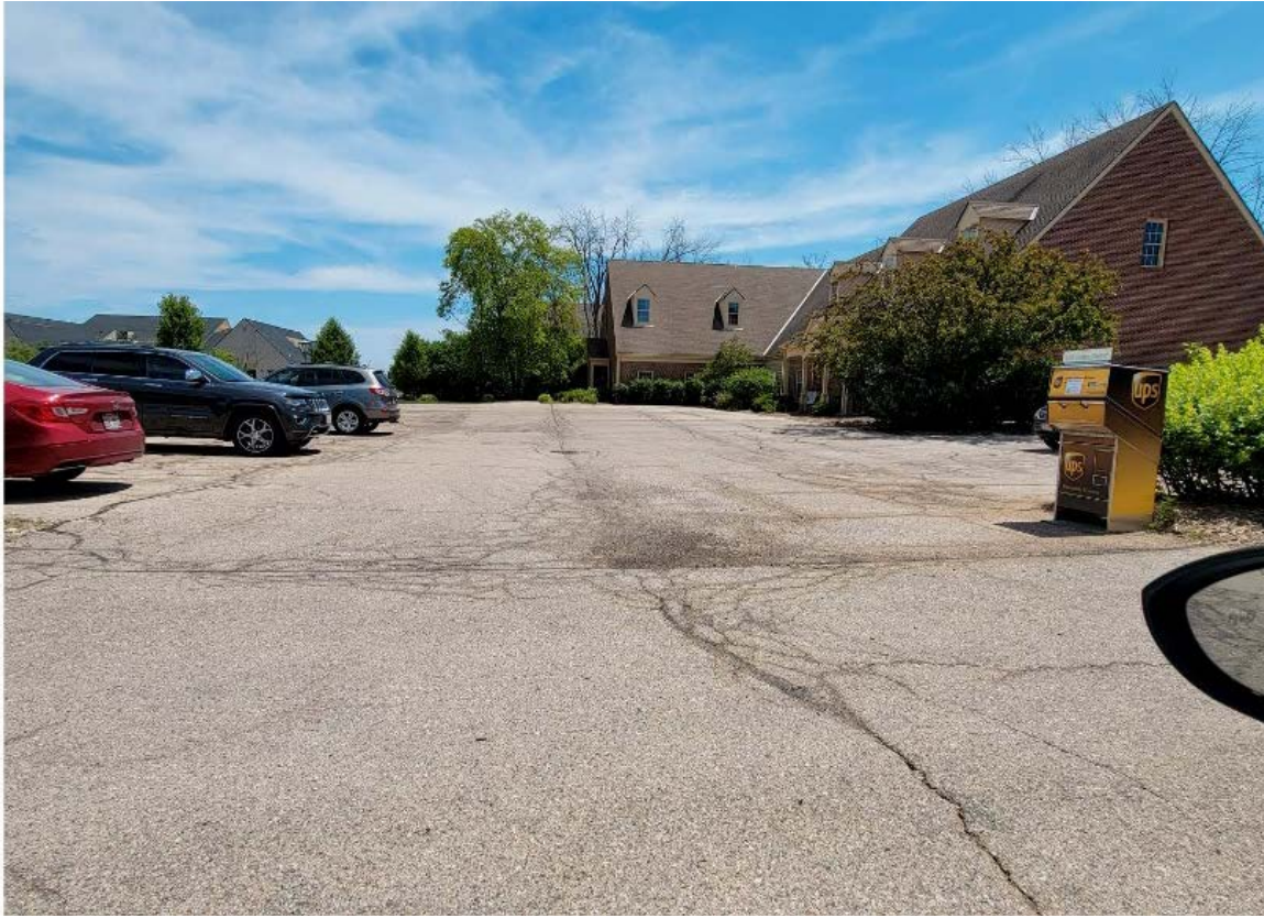
Exhibit 1: Deteriorated Parking Lot and overgrown/missing landscaping.
