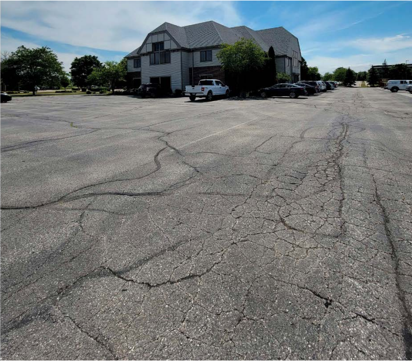
Exhibit 1: Deteriorating Parking Lot
