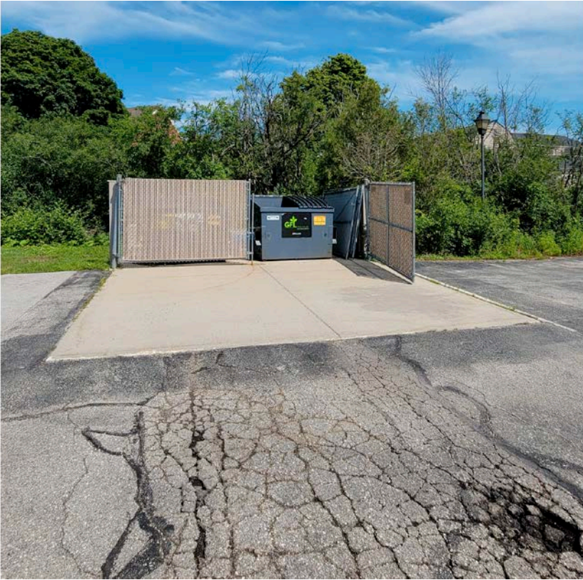
Exhibit 2: Dilapidated garbage enclosure with missing and broken walls
