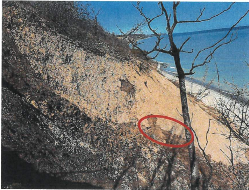
Photo 7: Looking north at the steep bare soil slope extending across the lower two-thirds of the bluff. Circled in red is a silt or sand seam visible on the bluff face.
