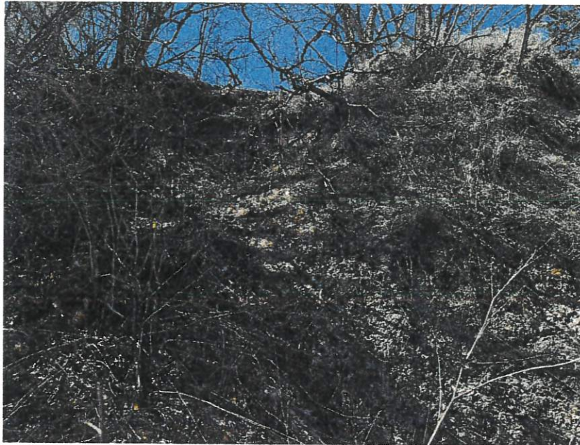
Photo 4: Looking west at the bluff face and steep scarps along the crest of the bluff.
