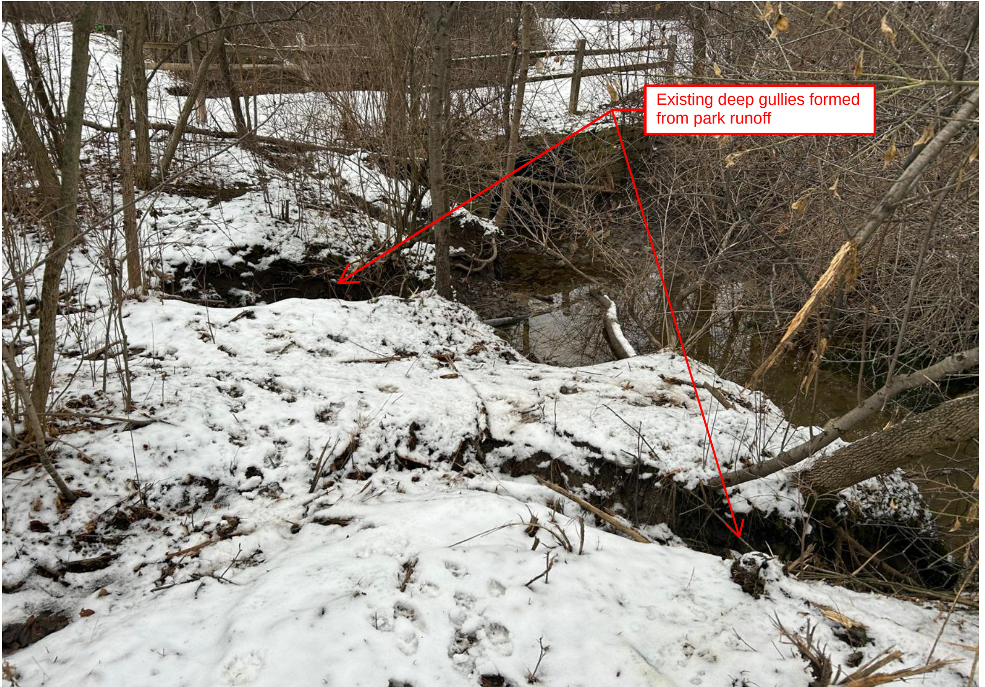
Katherine Kearney Carpenter Park – Gullies formed into bank of the main drainageway
